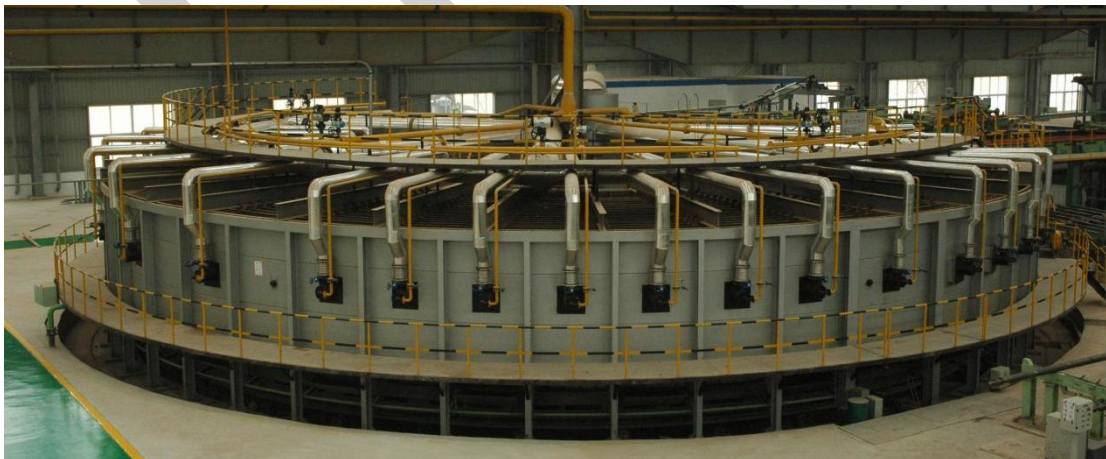
Heating furnace (Ring type)
