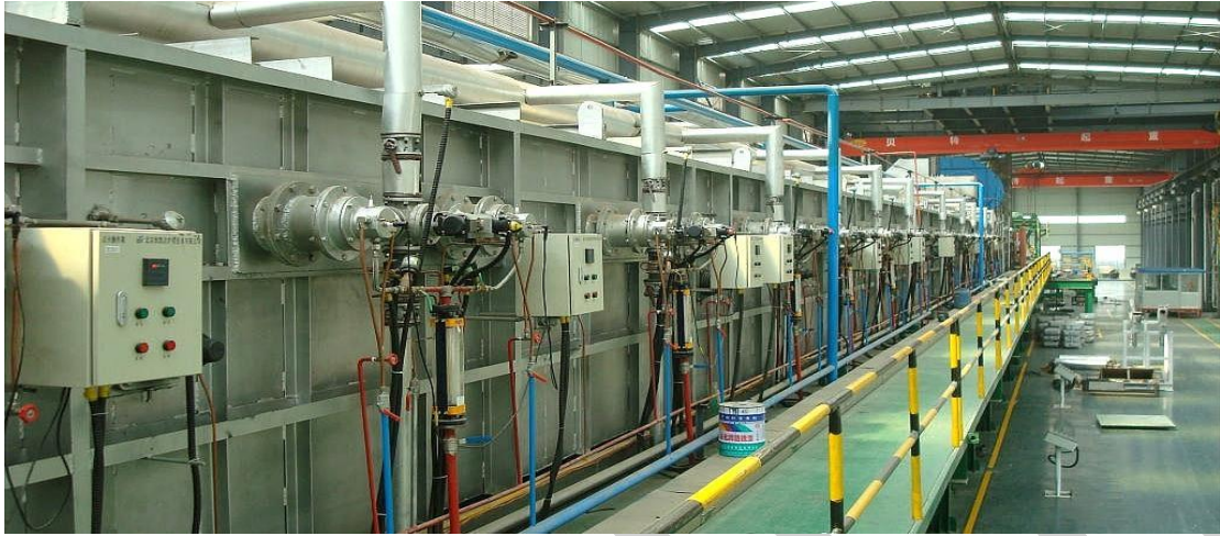
Annealing Furnace (退火炉)
