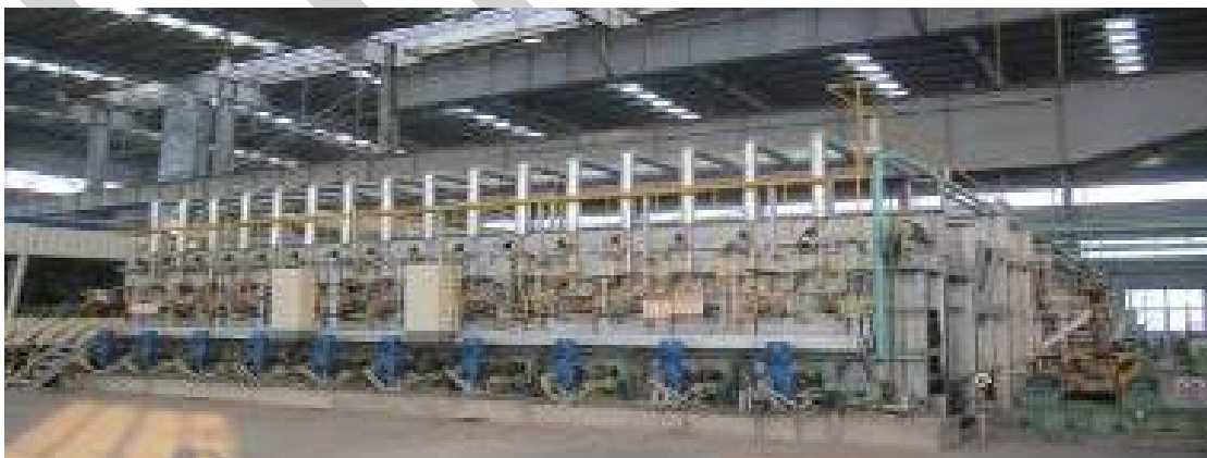
Quenching furnace(淬火炉)
